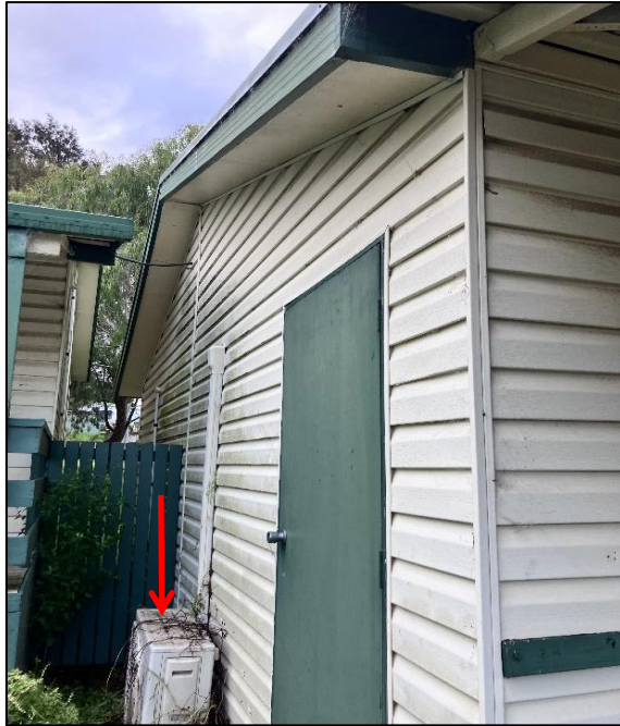
Photograph 5: B00T, exterior, roof, air conditioning unit, R410A, nil ODS identified.
