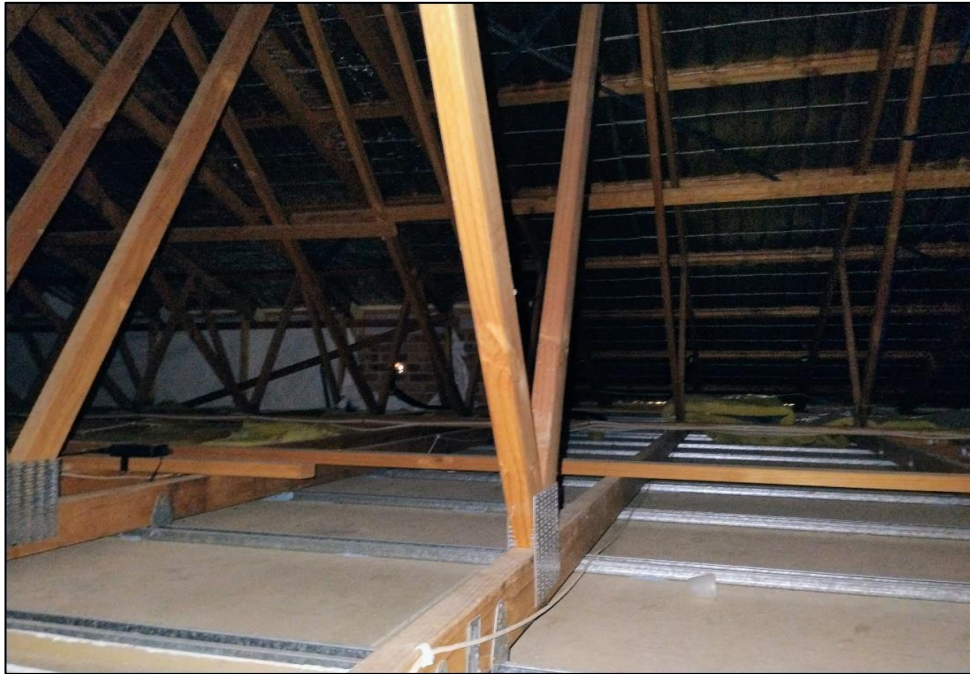
Photograph 9: B00E, ER0012, ceiling cavity, settled dust / debris, elevated lead concentration not identified.
