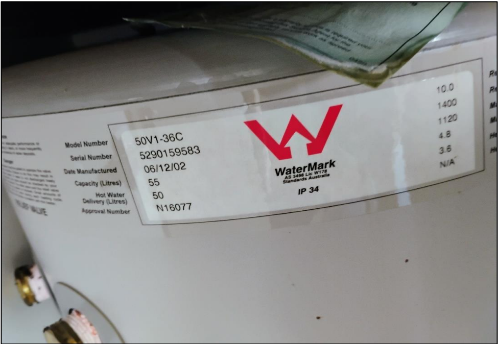
Photograph 11: B00E, ER0024, WaterMark hot water unit (circa 2002), insulation, SMF (suspected).
