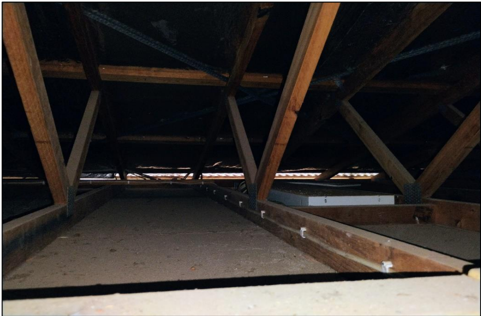
Photograph 6: B00T, rooms and areas in general, ceiling cavity, settled dust / debris, elevated lead concentration detected.
