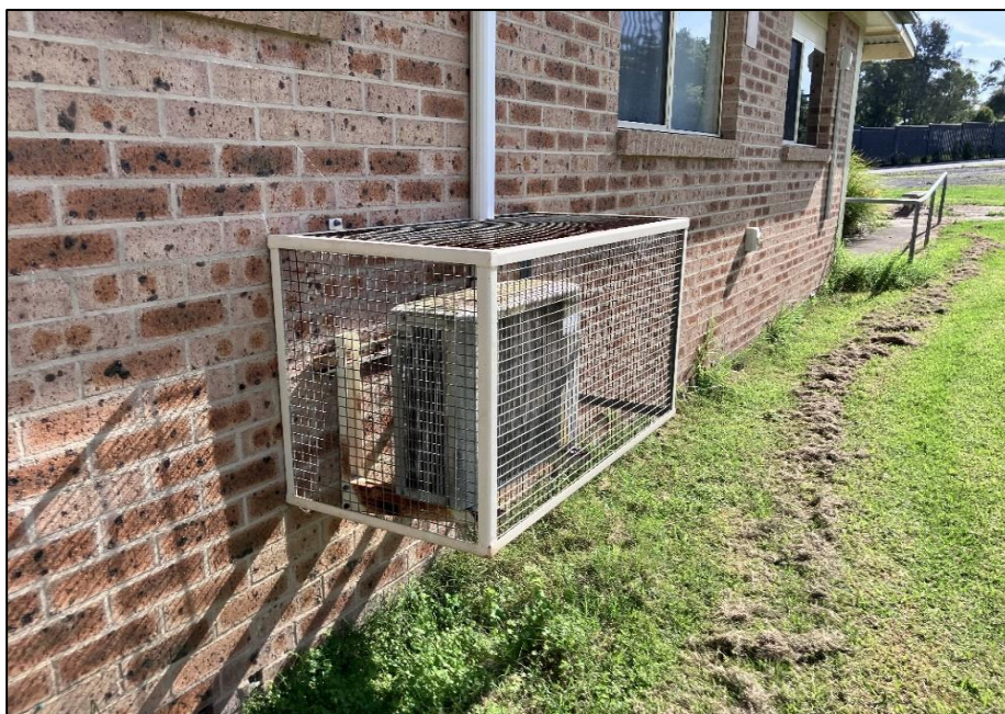
Photograph 16: B00W, exterior, southeastern façade, Fujitsu air conditioner, not determined, inaccessible / illegible compliance plate(s).
