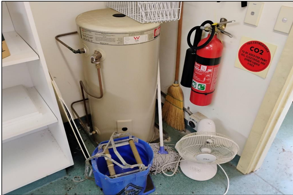
Photograph 7: B00U, UR0003, Dux hot water unit (circa 2001), insulation, SMF (suspected).
