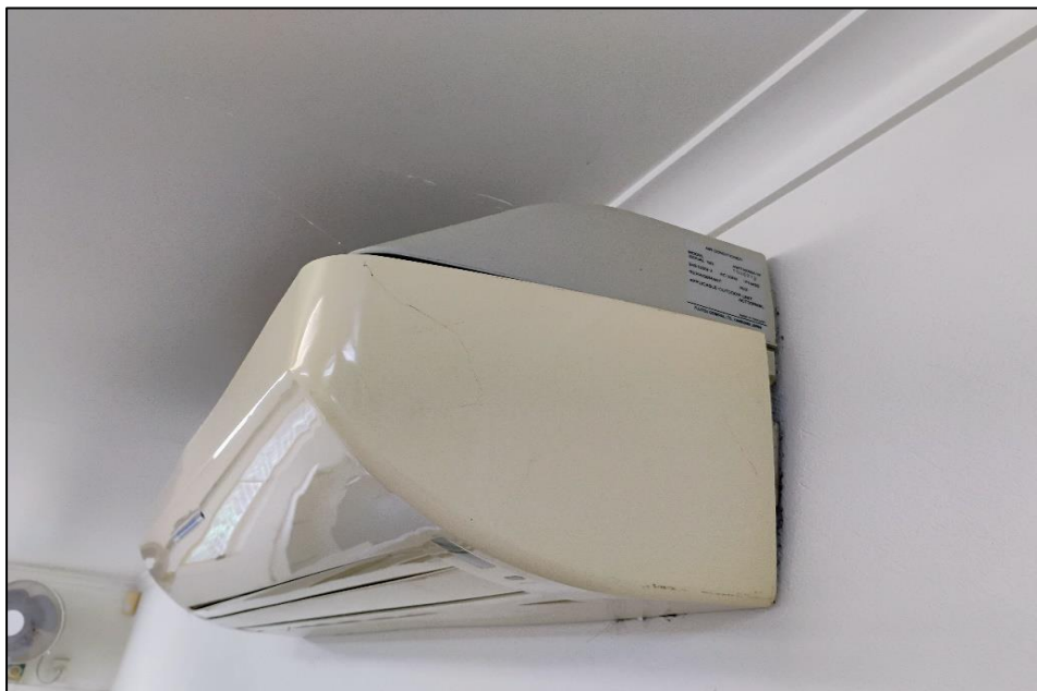
Photograph 9: B00U, exterior, roof, air conditioning unit(s), R22, ODS identified.
