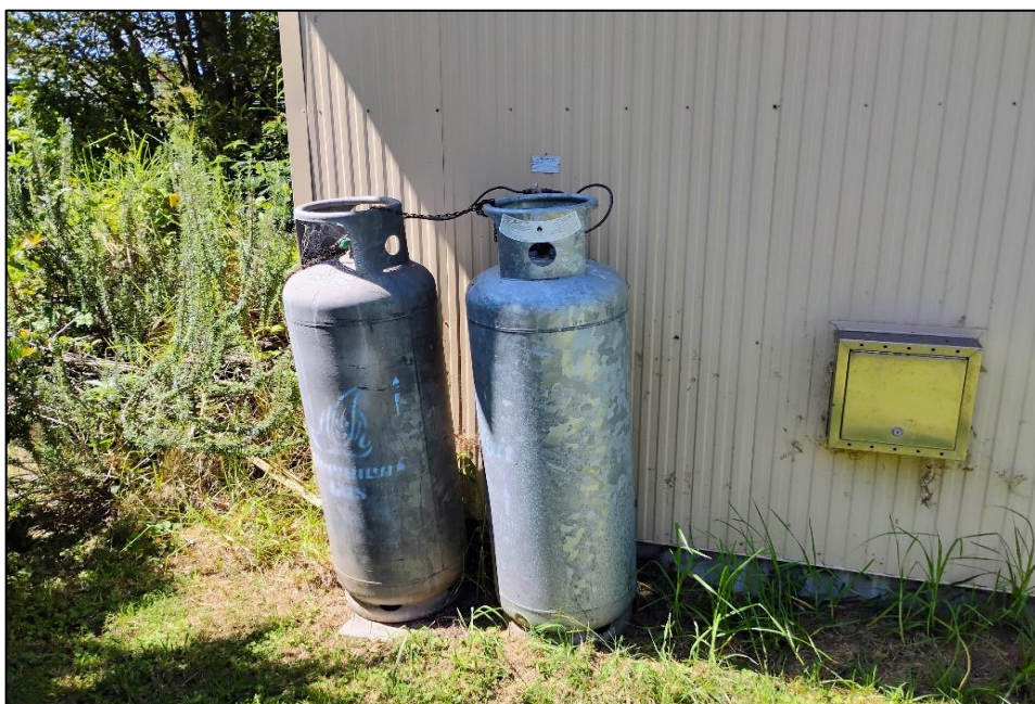
Photograph 8: B00H, exterior, designated LPG storage , LPG tanks (x2).
