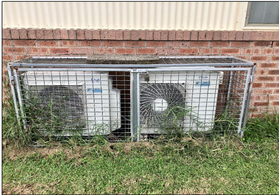
Photograph 9: B00V, exterior, western façade, north end, air conditioning units (x2), R410A, nil ODS identified.
