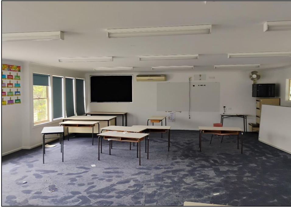
Photograph 7: B00Q, rooms and areas in general, fluorescent light fittings, internal components, nil PCB (suspected).
