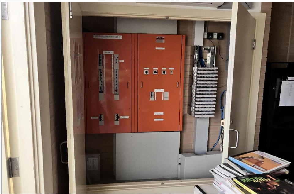
Photograph 6: B00B, BR0015, interior of electrical panel(s), materials in general, suspected non-asbestos.
