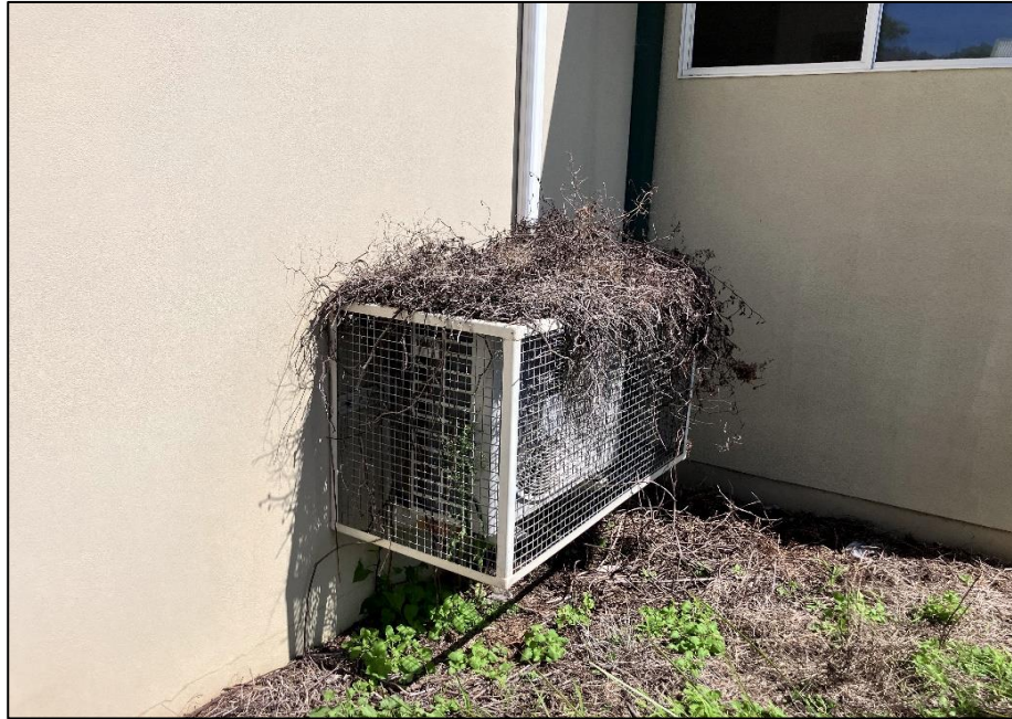
Photograph 19: B00W, exterior, northeastern façade, air conditioning unit, R410A, nil ODS identified.
