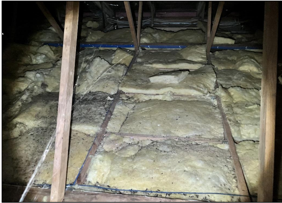
Photograph 13: B00W, ceiling cavity, top of ceiling, insulation batts, SMF identified visually.
