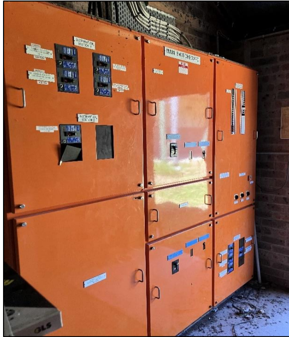
Photograph 9: B00W, WR0015, electrical cabinet(s), internal components, inaccessible.
