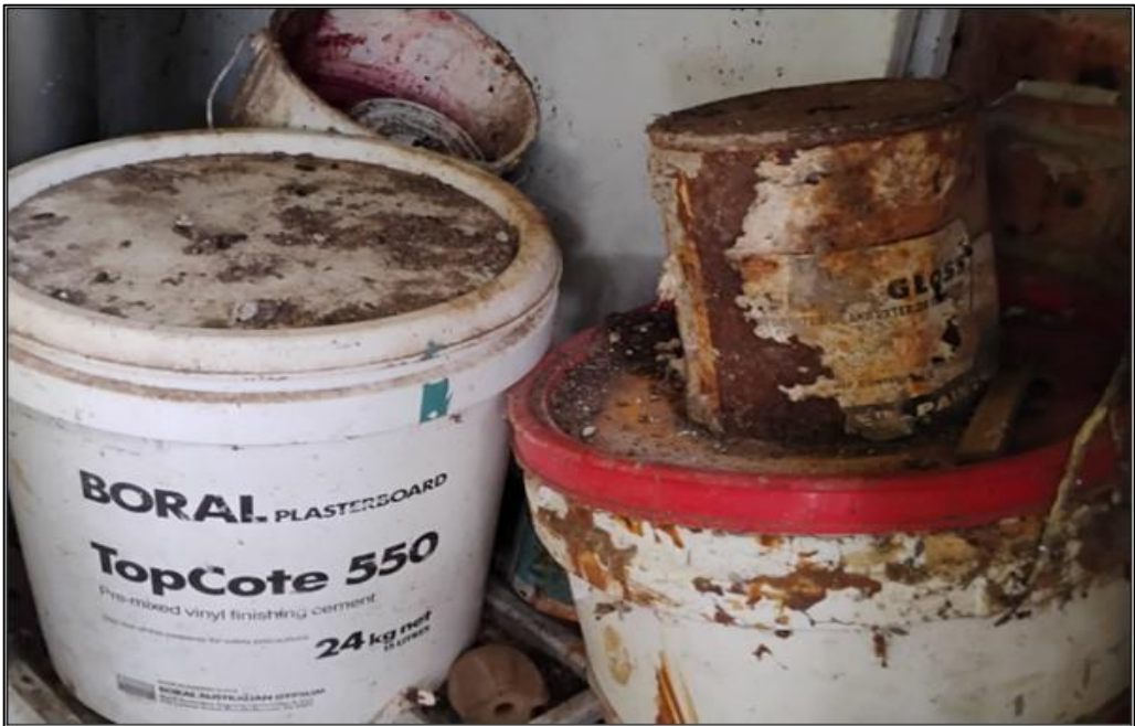
Photograph 4: B00P, sub floor area, general construction supplies/waste.
