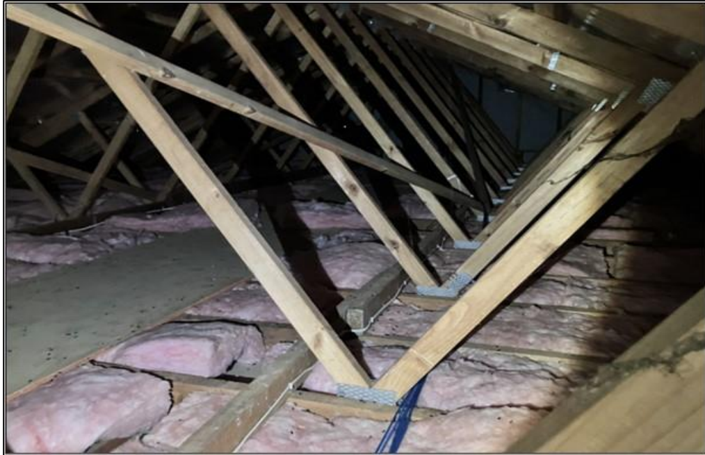
Photograph 5: B00P, ceiling cavity, top of ceiling, insulation (SMF identified visually).
