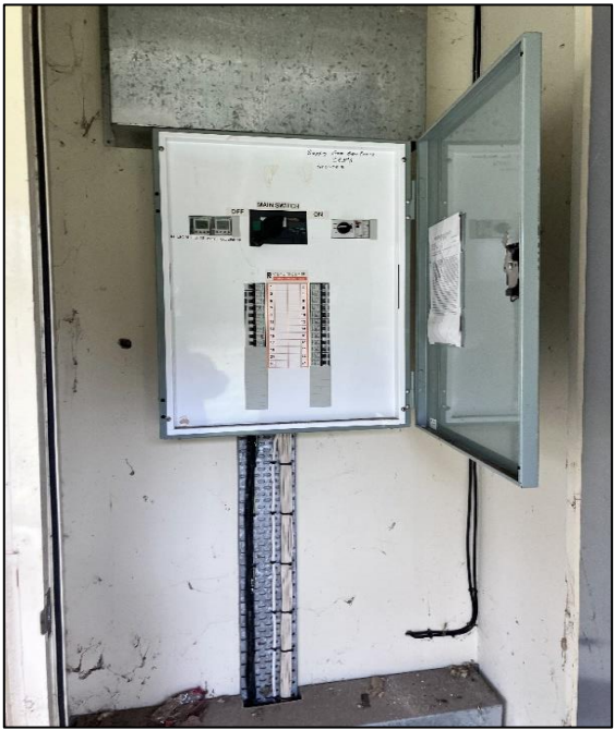
Photograph 4: B00V, interior, VR0009, within electrical panel(s), materials in general, inaccessible.
