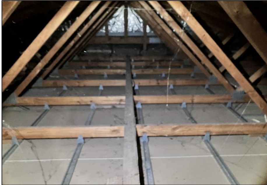
Photograph 7: B00C, interior, ceiling cavity, settled dust / debris, elevated lead concentration detected.
