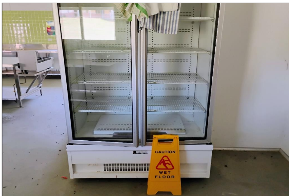
Photograph 7: B00H, HR0004, refrigerated display unit, unconfirmed, nil ODS suspected.
