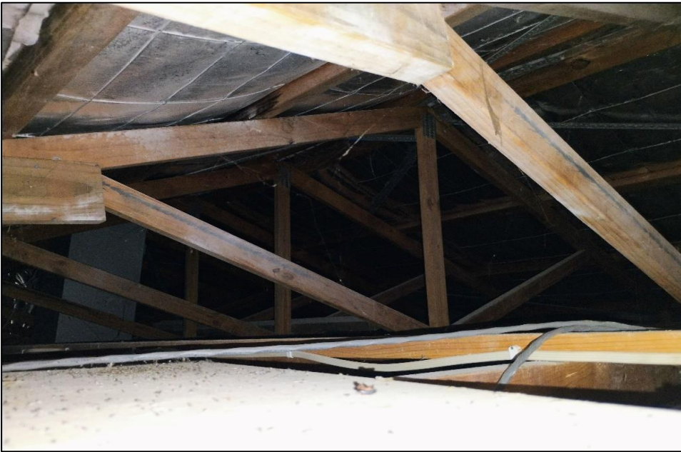
Photograph 6: B00U, rooms and areas in general, ceiling cavity, underside of roof, insulation, SMF identified visually.
