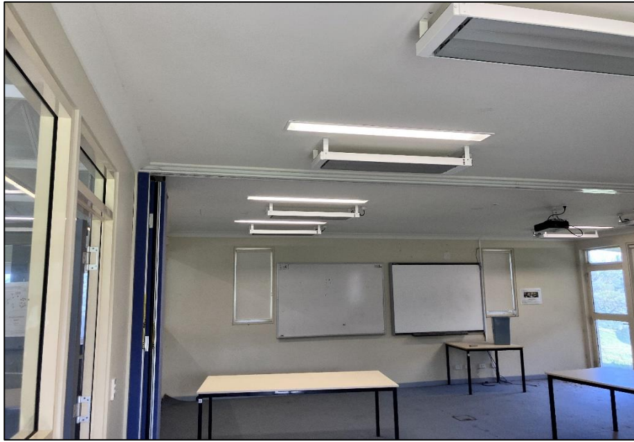
Photograph 7: B00V, rooms and areas in general, fluorescent light fittings, internal components, nil PCB (suspected).
