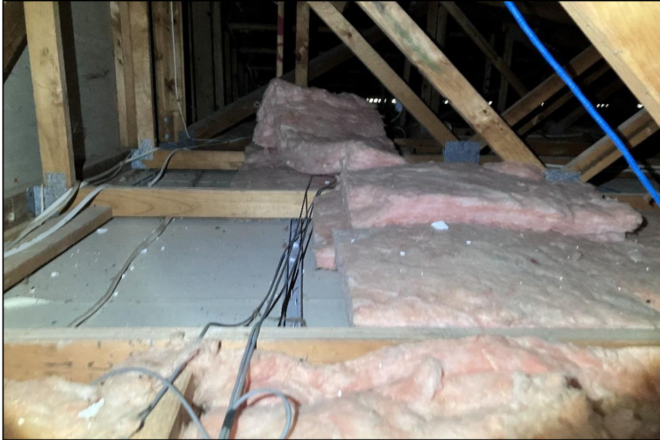
Photograph 9: B00A, ceiling cavity, settled dust / debris (elevated lead concentration detected) and insulation to top of ceiling (SMF).
