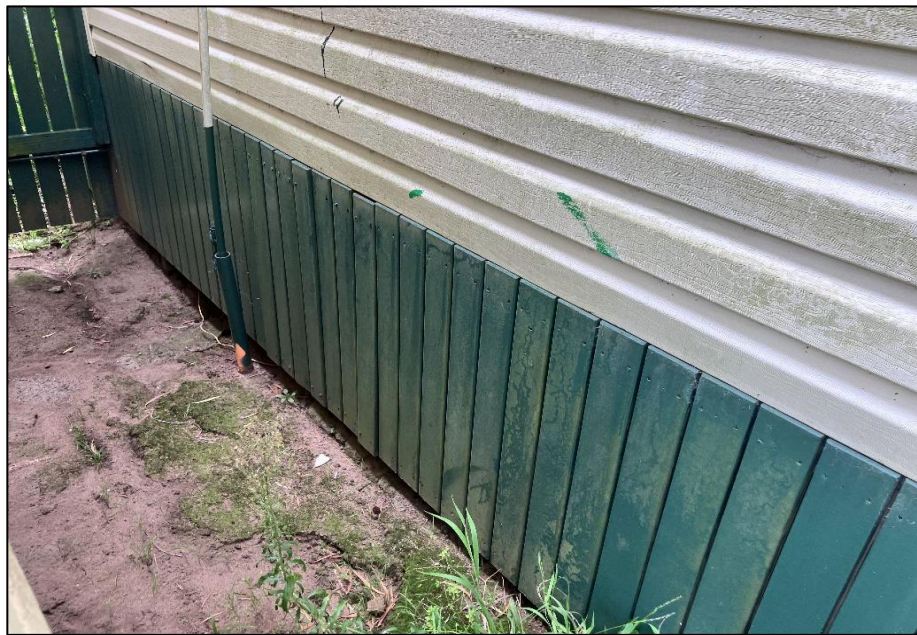
Photograph 2: B00S, exterior, subfloor area, materials in general, inaccessible.
