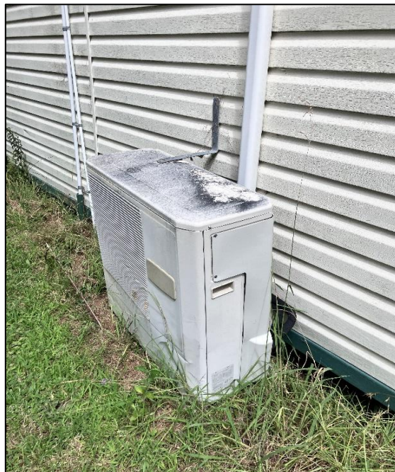
Photograph 8: B00S, exterior, air conditioning unit, R22, ODS identified.
