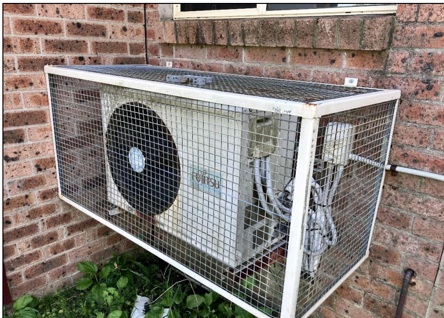
Photograph 17: B00W, exterior, southwestern façade, Fujitsu air conditioner, R22, ODS identified.
