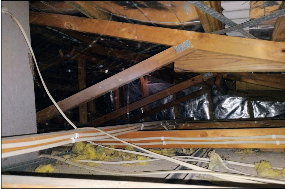
Photograph 5: B00U, rooms and areas in general, ceiling cavity, settled dust / debris, elevated lead concentration detected.
