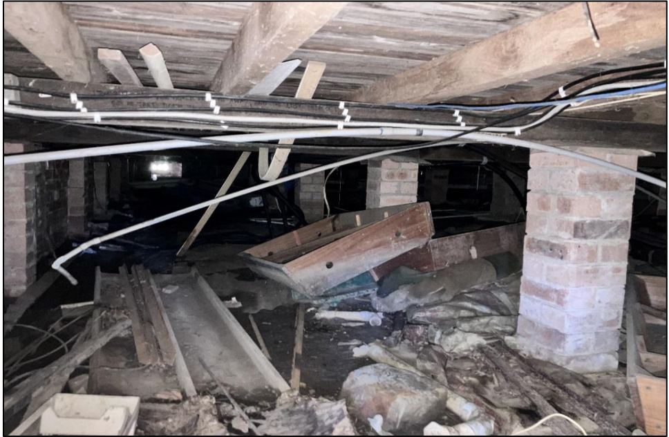
Photograph 11: B00W, subfloor, throughout, materials in general, limited / restricted access.
