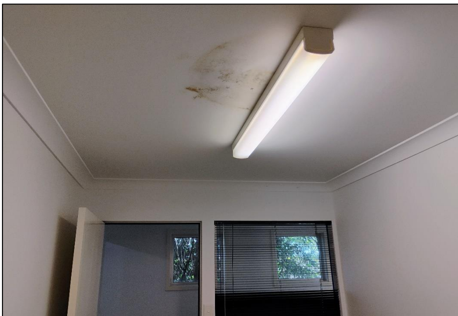
Photograph 15: B00W, rooms and areas in general, fluorescent light fittings, internal components, nil PCB (suspected).
