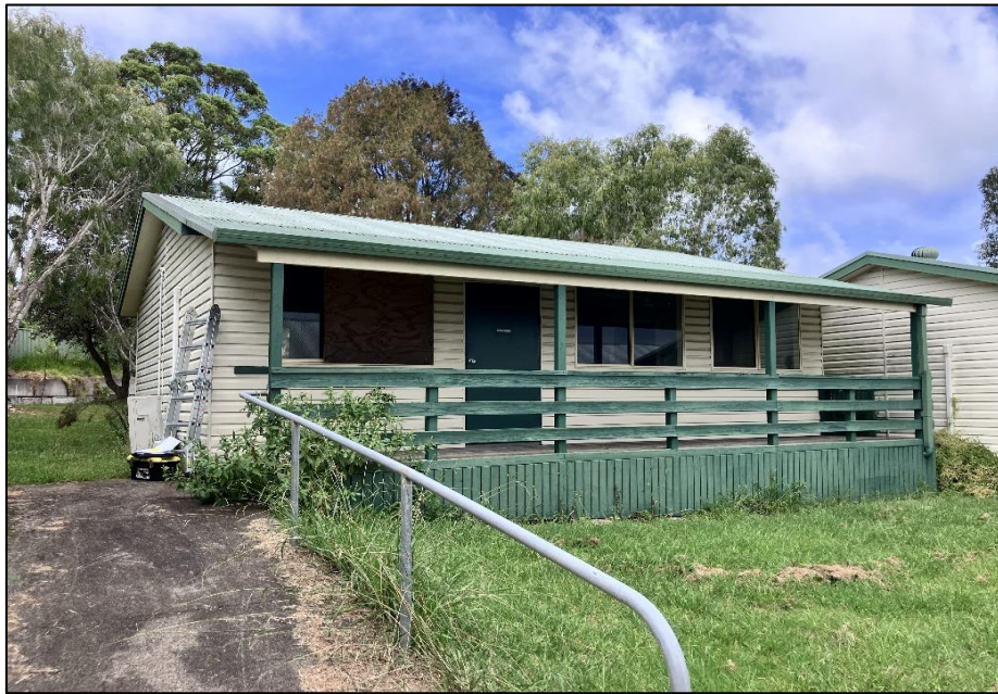
Photograph 3: B00S, exterior, front deck, timberwork, green paint.
