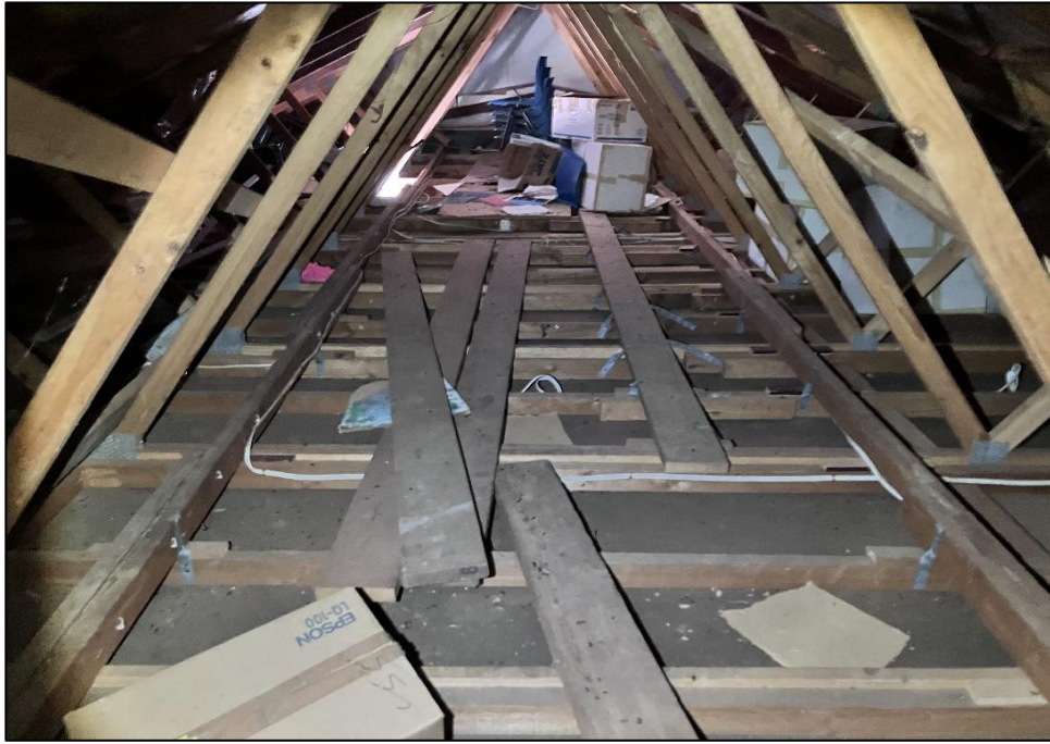
Photograph 5: B00Q, QR003, ceiling cavity, settled dust / debris, elevated lead concentration not identified.
