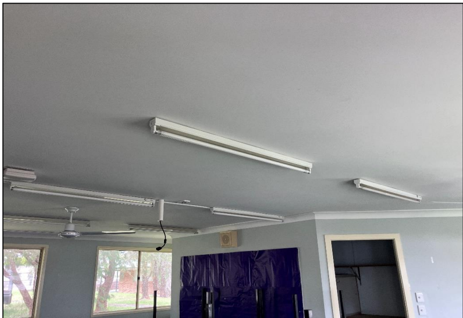
Photograph 6: B00S, rooms and areas in general, fluorescent light fittings, internal components, nil PCB (suspected).
