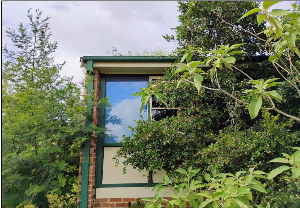
Photograph 1: B00P, exterior, west façade, infills, eave linings, fibre cement sheeting, no asbestos detected by analysis.
