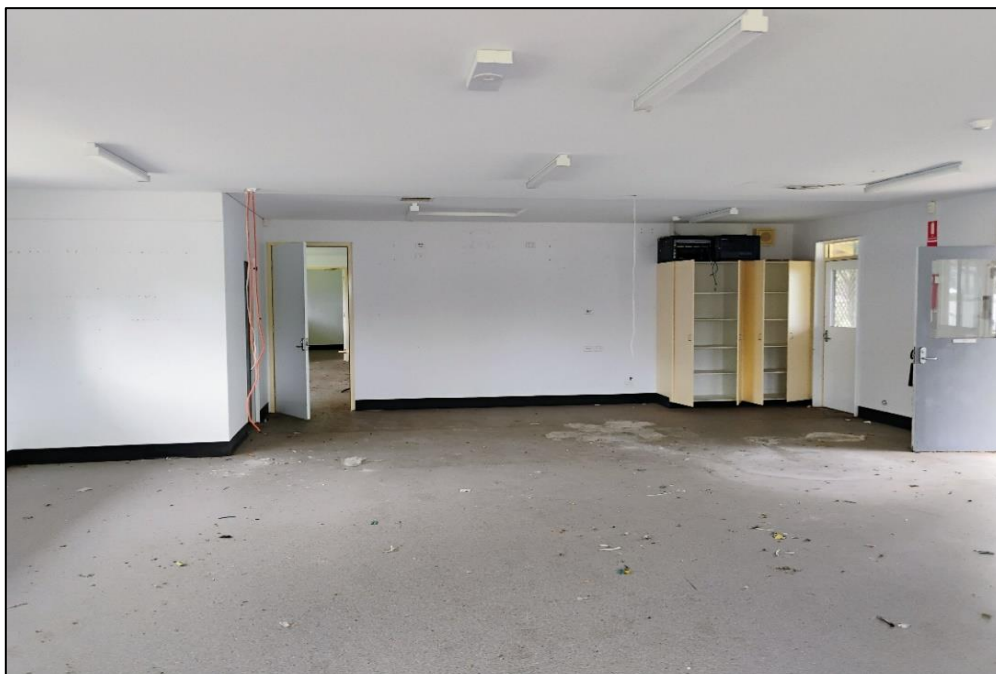
Photograph 7: B00D, rooms and areas in general, fluorescent light fittings, internal components, nil PCB (suspected).
